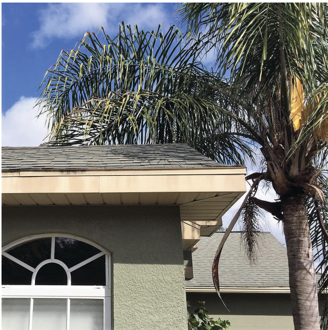
Figure 5. Palm leaves should be removed if hanging over a roof.
