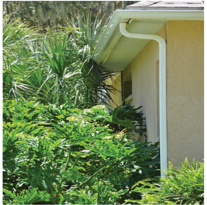
Figure 7. Overgrown plants allowing access to the roof.
