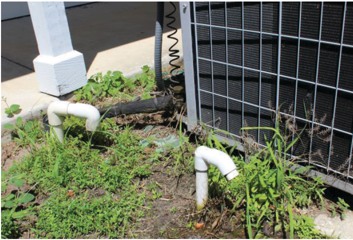
Figure 13. A/C lines should be directed away from the foundation. Credits: Brooke Moffis, UF/IFAS
