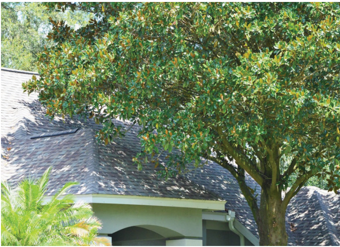
Figure 4. Tree limbs touching the roof can provide access to rodents and other pests.
