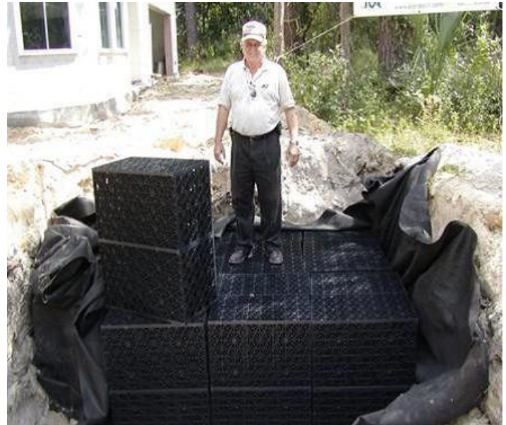
Figure 4. A subsurface exfiltration system installed at the Madera subdivision in Gainesville, FL. Credits: Program for Resource Efficient Communities, University of Florida 2004
