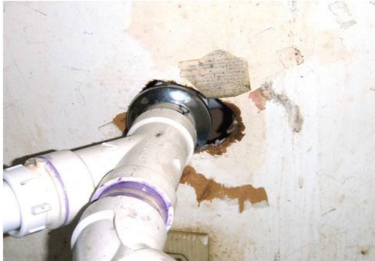
Figure 2. An improperly installed escutcheon plate can be repaired by the DOHRE Maintenance Section.
