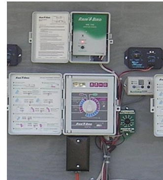
Figure 2. Four brands of soil moisture sensor controllers with an electronic time clock. Credits: Michael Dukes.
