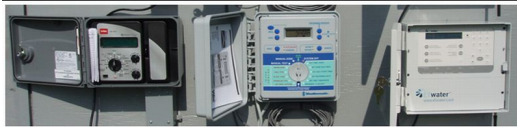
Figure 1. Photo of three brands of ET controllers undergoing testing at the University of Florida, Agricultural and Biological Engineering Department. Credits: Stacia Davis.
