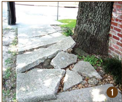
Figure 1 Sidewalk located too close to the root flare of a large tree.
