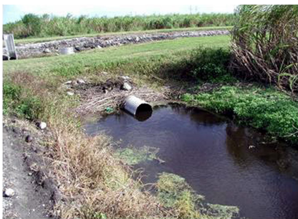
Figure 9. Raised culvert bottom reduces bedload sediment transport.
