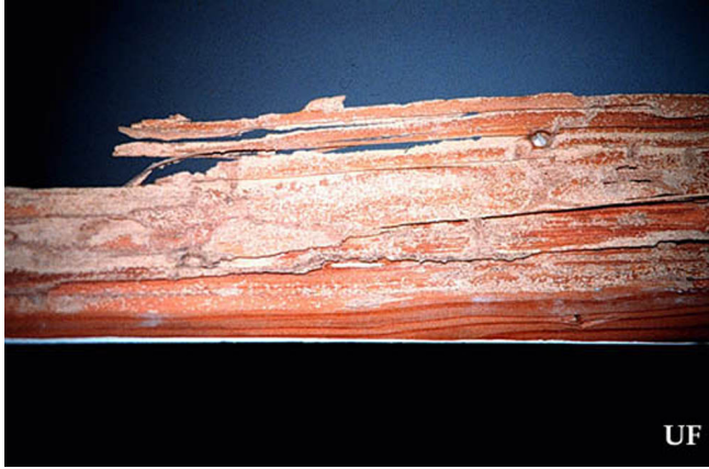
Figure 9. Damage and fecal spotting by Heterotermes subterranean termites to wood molding, Miami, Florida.
