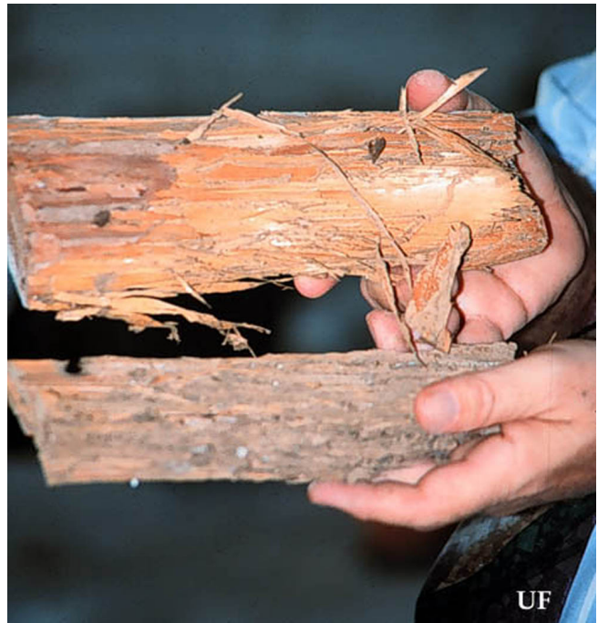
Figure 11. Heterotermes subterranean termite damage showing dry and shredded appearance of wood, Miami, Florida. Credits: Rudolf H. Scheffrahn, University of Florida
