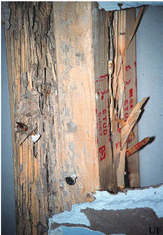
Figure 10. Damage and fecal spotting by Heterotermes subterranean termites in dry framing, Miami, Florida. Credits: Rudolf H. Scheffrahn, University of Florida
