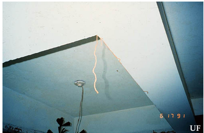
Figure 12. Heterotermes subterranean termite foraging tube dropping from living room ceiling, Santo Domingo, Dominican Republic. Credits: Rudolf H. Scheffrahn, University of Florida
