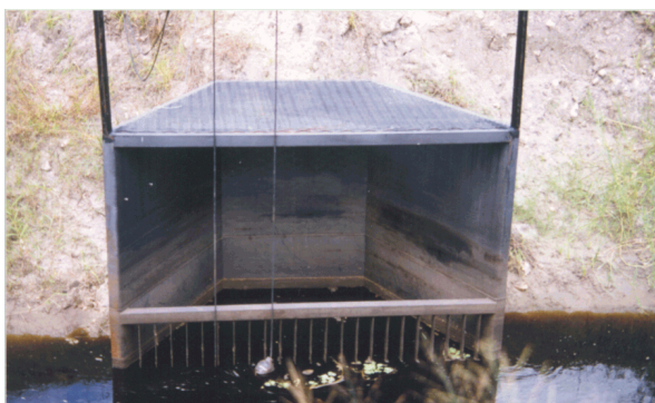
Figure 9. Float controls for drainage pump.
