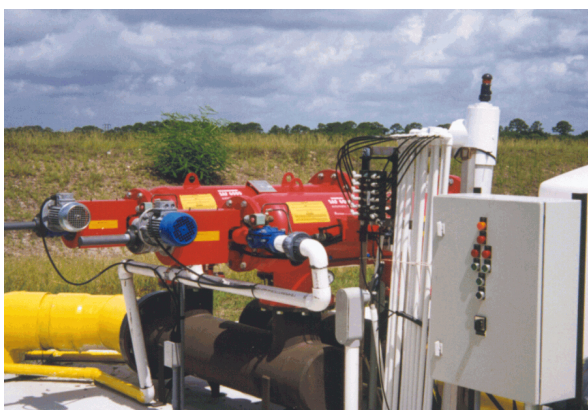
Figure 7. Control panel for automatically backflushing filters based on pressure differential between inlet and outlet of filter.
