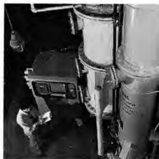
Pilot Scale Ion Exchange Columns
