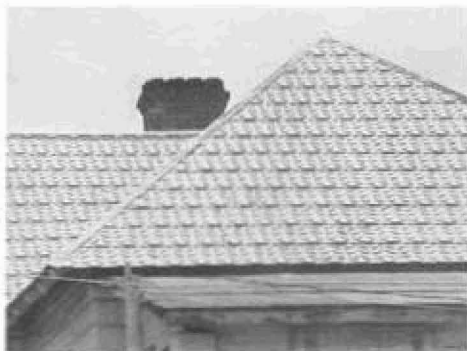
The district's Reed Bryan House retains its unusual roof of patterned metal, typical of many structures built shortly after the turn of the century in south Florida.
