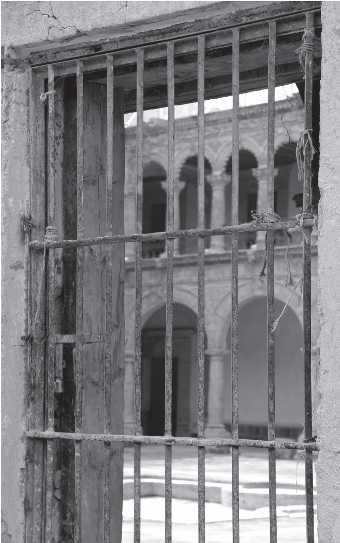
Figure 5. Detail of the decay in one of the outer windows of Claustro de la Merced, c. 1676-1703, Mexico City, Mexico. Photo credit: Martha Lara Vázquez.
